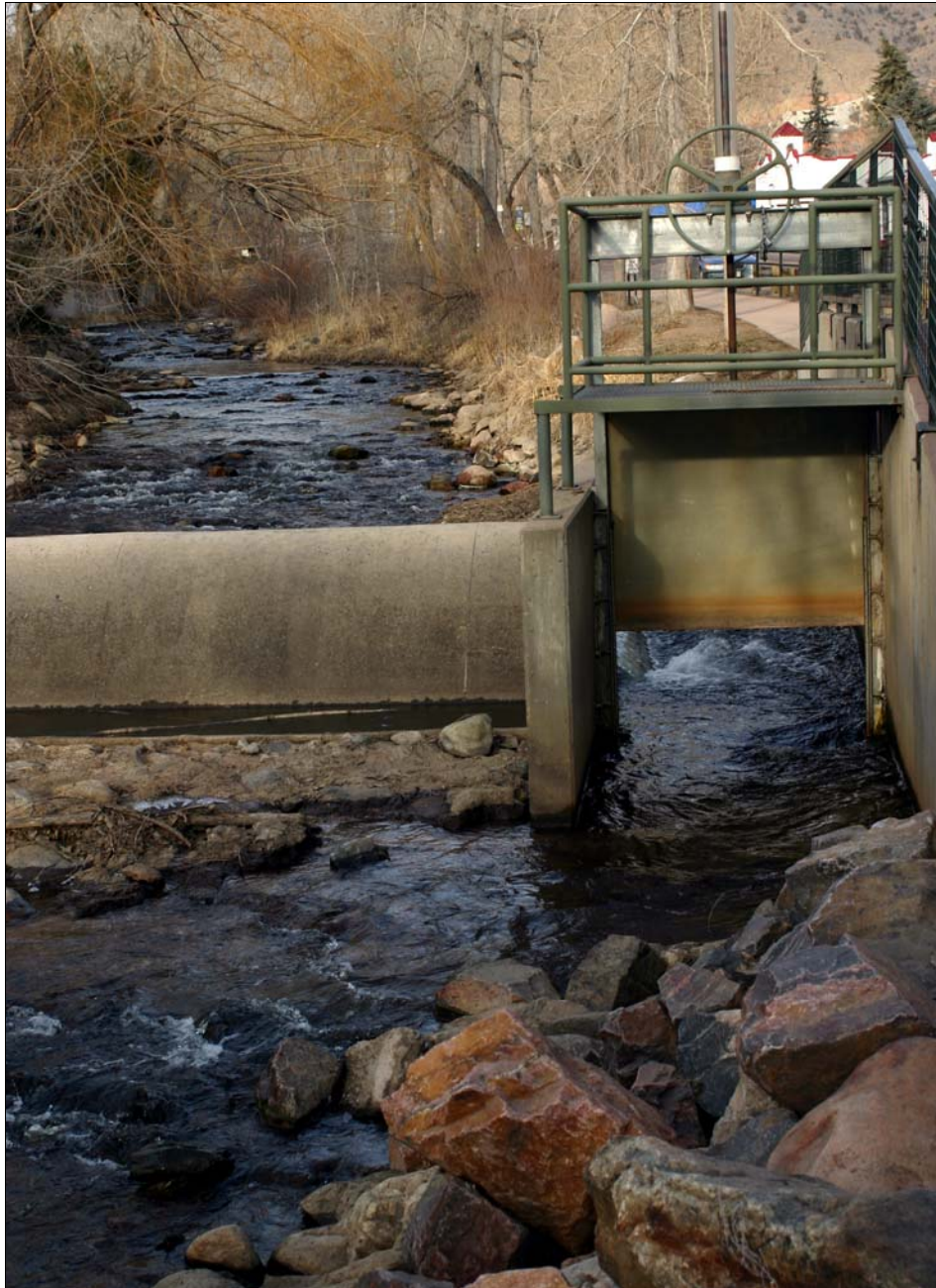
Diversion structure on Bear Creek near Morrison for the Harriman Ditch and the Warrior Ditch
