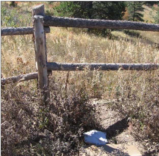
Typical well head with vault and electrical panel
